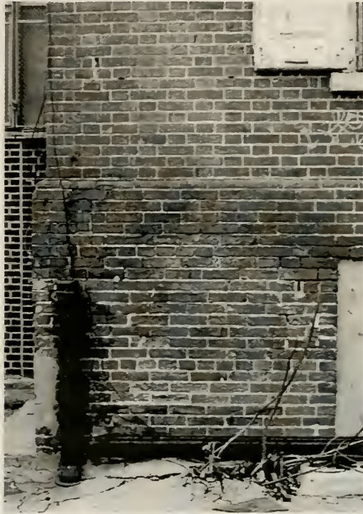
Figure 23 Missing Downspout. Ground Conditions and Masonry Saturation, 1998 Photograph by Author
